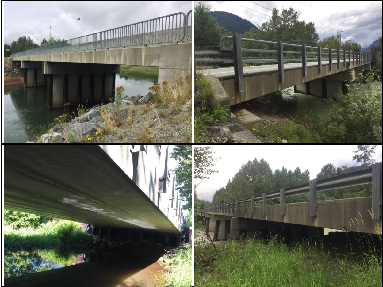
Figure 9. Bridges in the Pemberton area used by bats during the summer of 2019.
